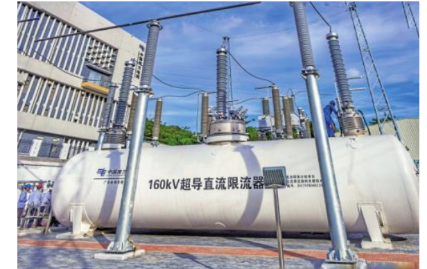
the World's first 160kV DC SFCL
