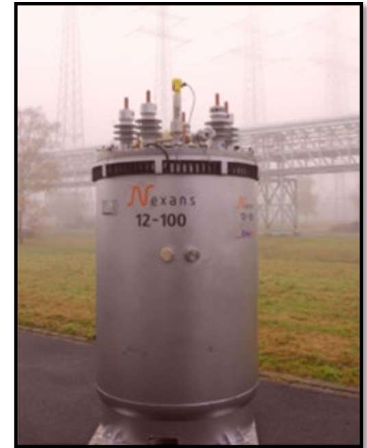
Superconducting Fault current limiters (SFCL)
