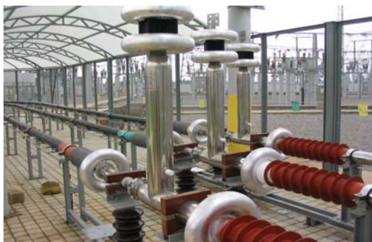
Fig.9. The 33m long, 35 kV/2.0kA HTS AC cable installed in Puji substation.
