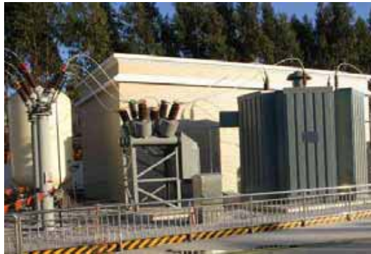
Fig.13. The 35kV/1.5kA core-saturated type SFCL at the Puji substation.
