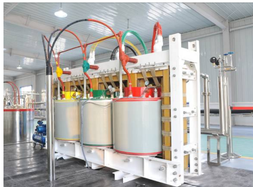
Fig.14. The 630 kVA three-phase HTS Transformer.
