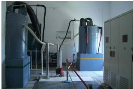
Fig.12. The 10.5kV/1.5kA SFCL installed at Loudi Substation.
