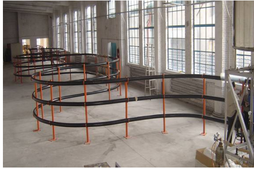
Fig.10. The 75m long 10.5 kV//1.5kA HTS AC cable installed in Baiyin Changtong Cables Company.
