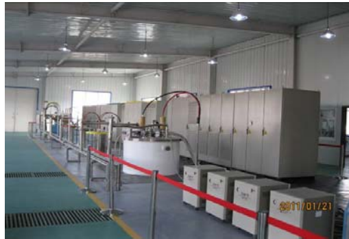
Fig.15. The 1MJ/0.5MW Superconducting Energy Storage Device.
