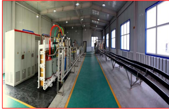
Fig.17. The 10.5kV Baiyin Superconducting Power Substation.
