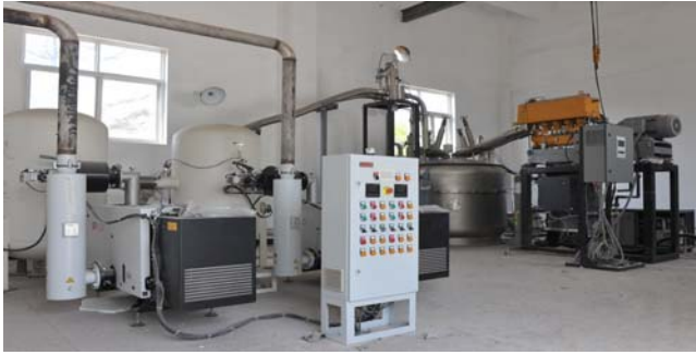
Fig.3. The refrigeration system for the 360m/10kA HTS DC cable.
