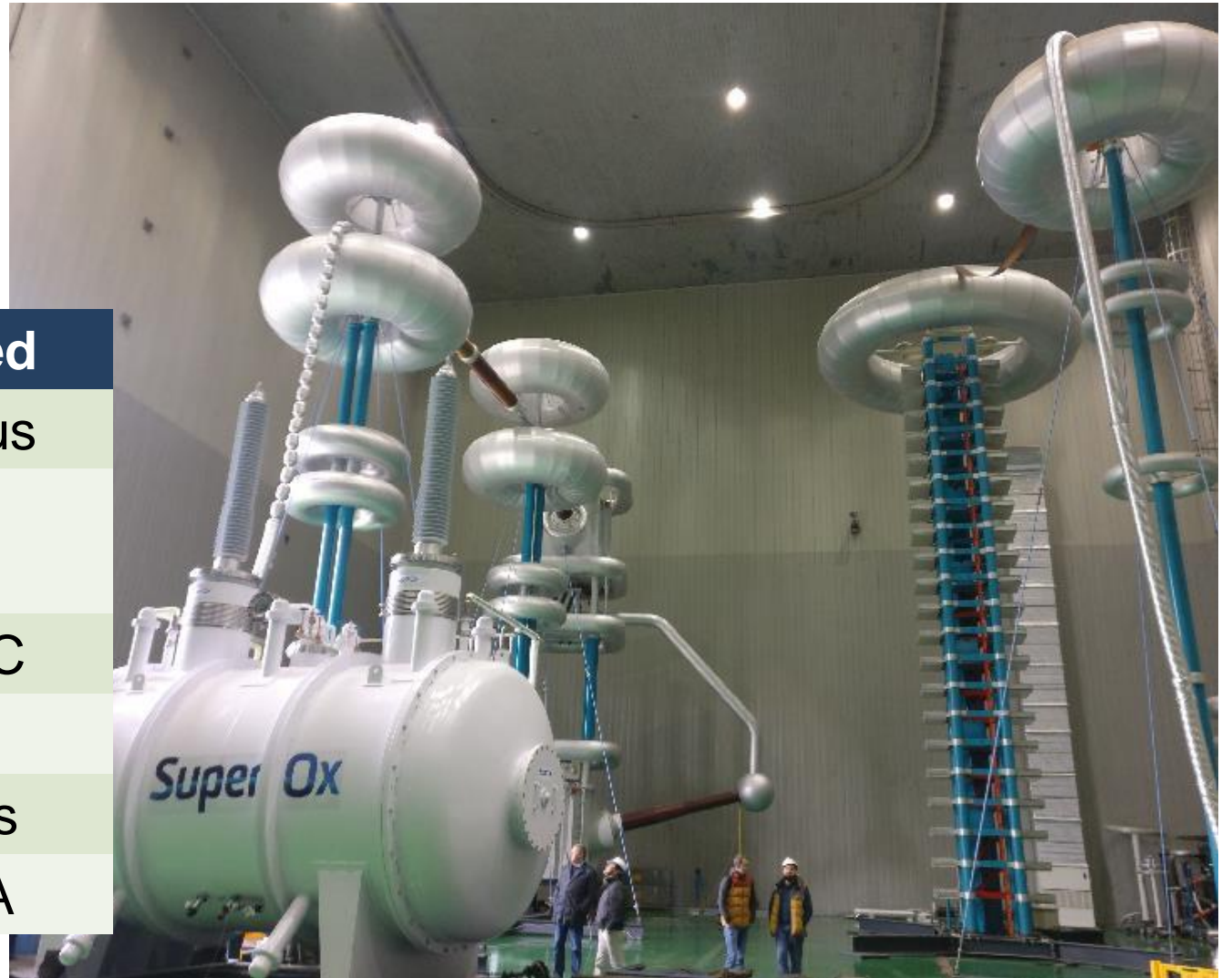
220 kV SFCL phase at the test site in KERI (Korea)
