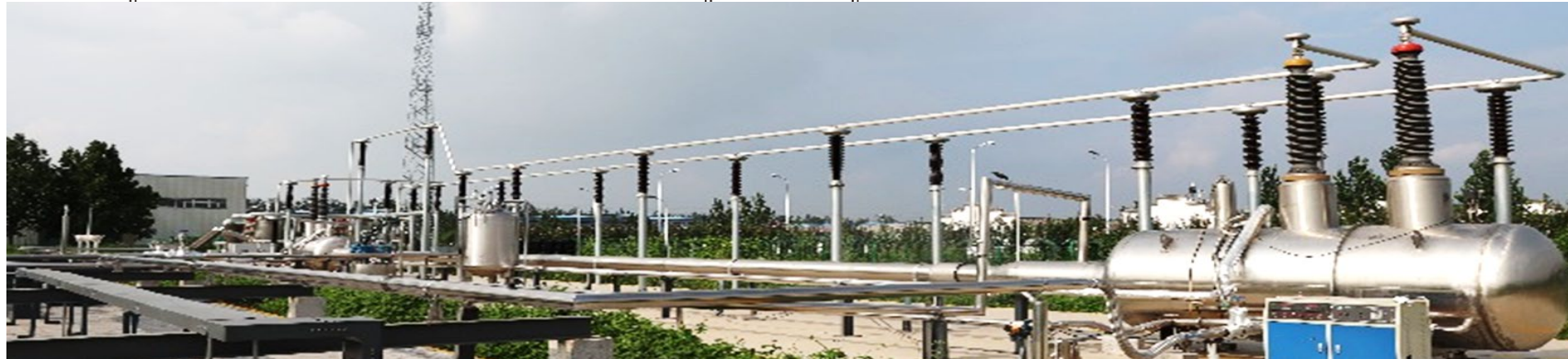
30m, \pm 100 kV/1 kA Superconducting Energy Pipeline tested at Langfang
