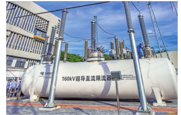
World's first 160kV DC SFCL
